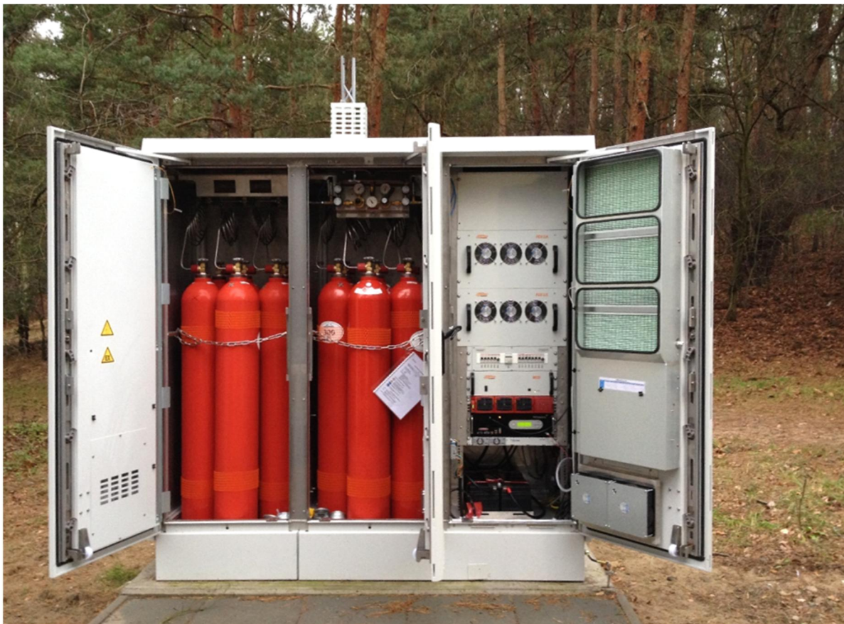
Figure 3-6: Example of a hydrogen-powered FC UPS
