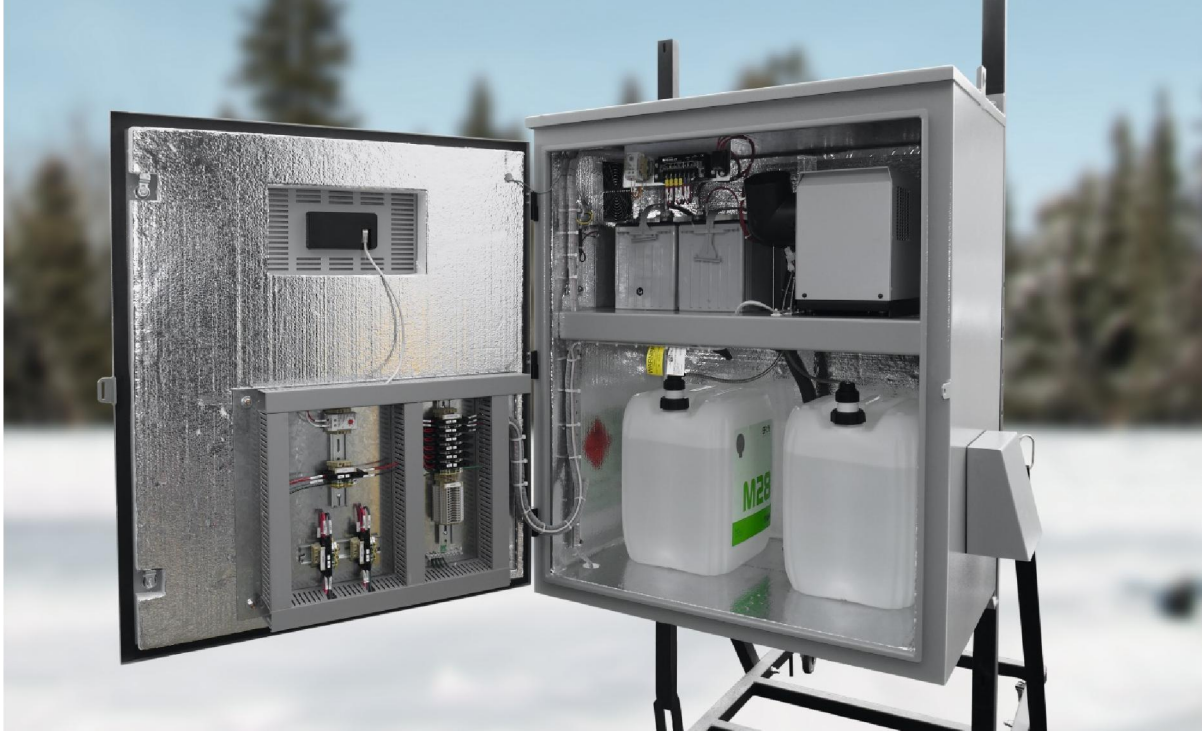
Figure 3-7: Example of a methanol-powered FC back-up power supply system
